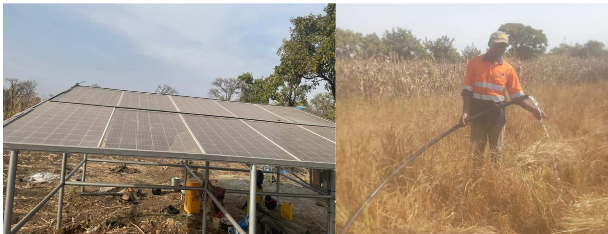
Installation of a Solar Powered Borehole at 20-acre Model Garden Farm in Balungu
